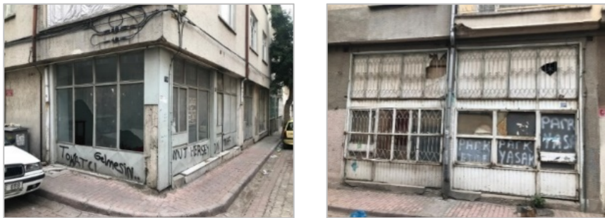
Figure 9. Vandalism acts in the area
